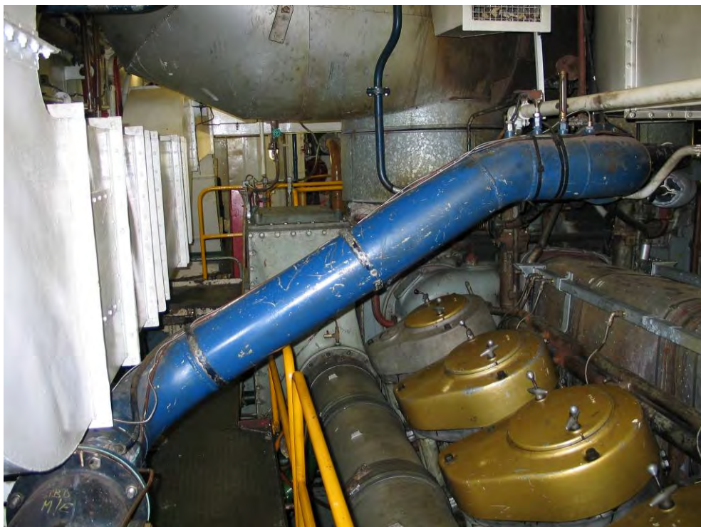
HMAS SUCCESS – Main Engine showing Jacket Water Cooling pipe work (blue)
