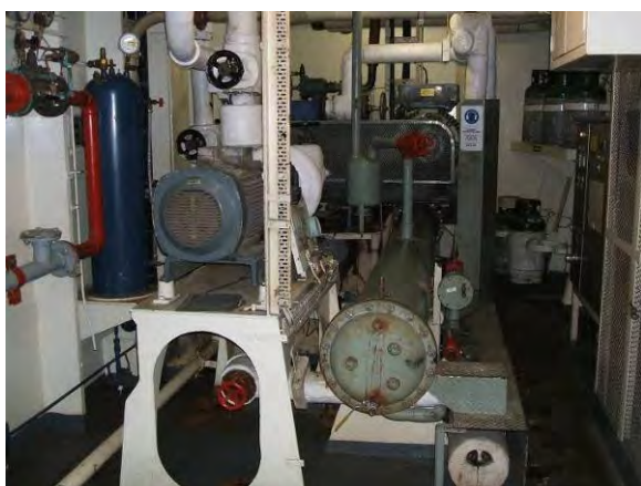
Current Forward Air Conditioning Unit
